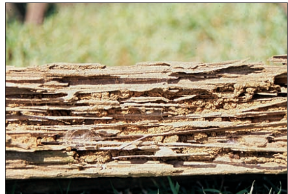
Figure 6. — Wood damaged by subterranean termites.
